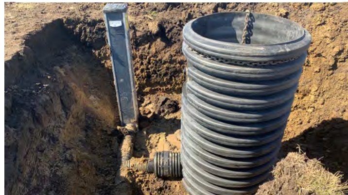
Figure 3. Gate Structures to Control Water Table
